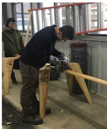
SUNY Geneseo students Brian Zapfel and Hiina Asami work on the construction of the Chimney Swift artificial nesting tower.
